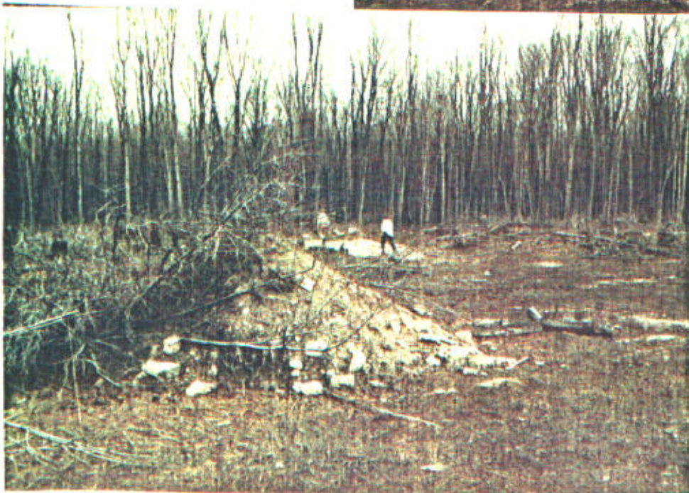
Fill and brush associated with USDA Forest Service construction of radio tower complex.
