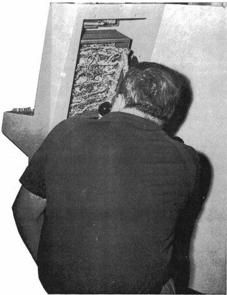
STUDYING A MASS of wiring in a 305 Switching Console is Earl Dunn, Switchman, Southern Bell, as he maintains one of the System's Consoles in the NORAD Control Center.
