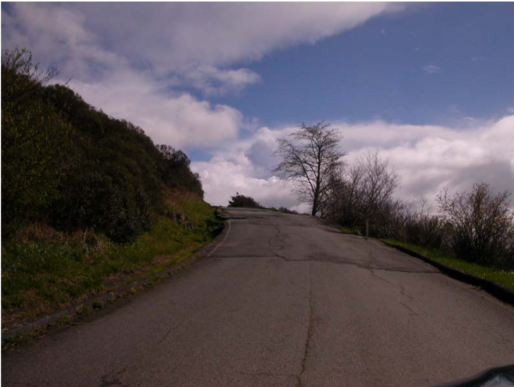
Figure 16 An example of site instability - roadways are subsiding throughout the property
