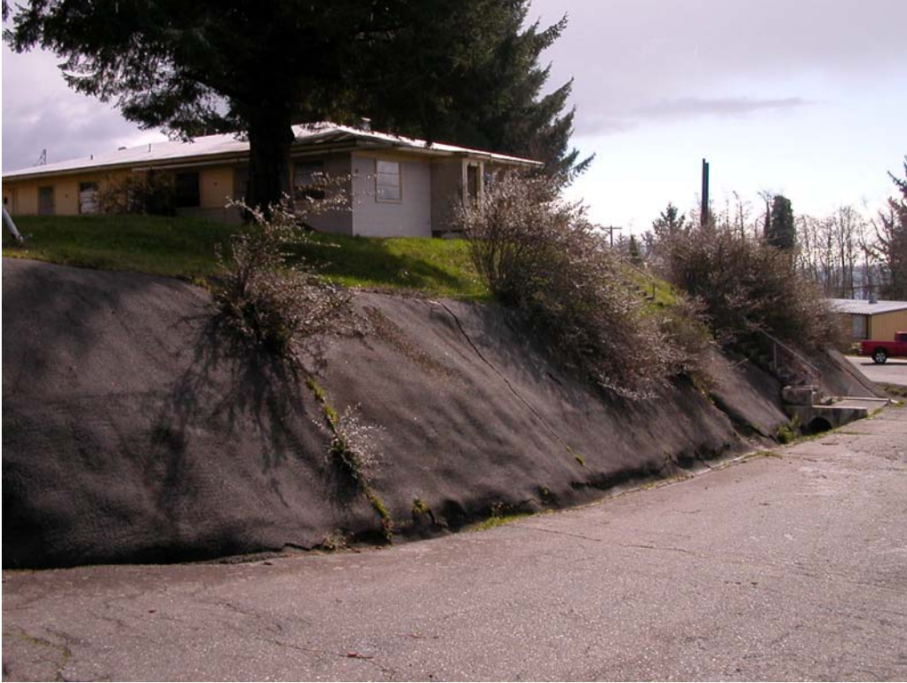
Figure 7 Building 108, as well as cracking hillslope stabilization material
