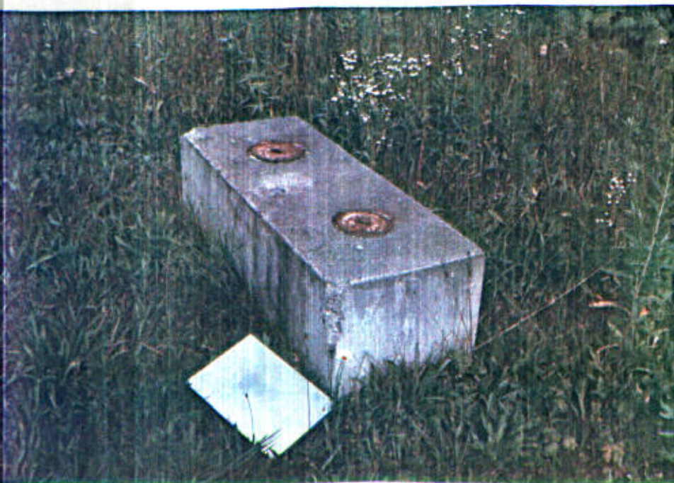
Underground fuel tank ports.
